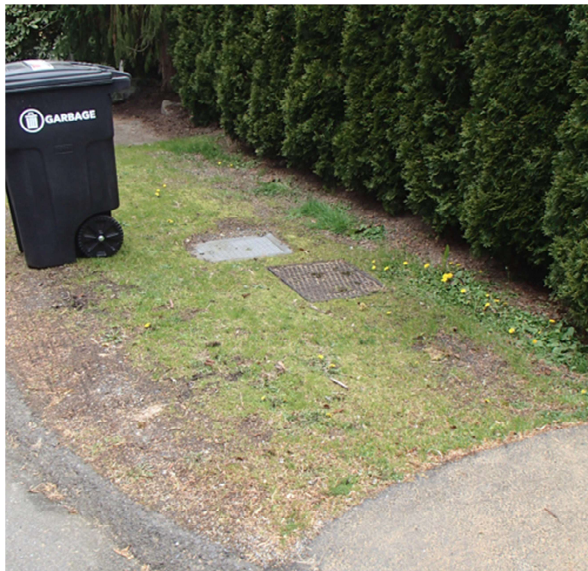
Photo No. 6 Looking northwesterly at CB 30a-25 (solid cover) where the SD crosses to the south side of the street and connects to CB 30a-34.
