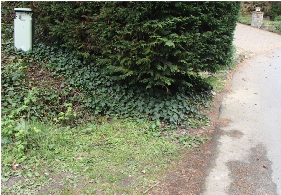
Photo No. 11 Looking southerly at CB #30a-37 just south of House #7820. Note ivy overgrowth but CB appears to be draining. Minor indication of erosion at the pavement edge. Inlet in street appears to be full of sediment (CB#30a-43) not on main line, so no impact to conveyance capacity.
