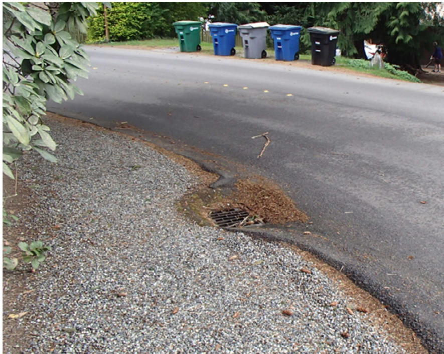
Photo No. 8 Looking southerly at CB #30a-51 opposite House #6035. Note accumulation of fir needles, but still appears to be draining well.
