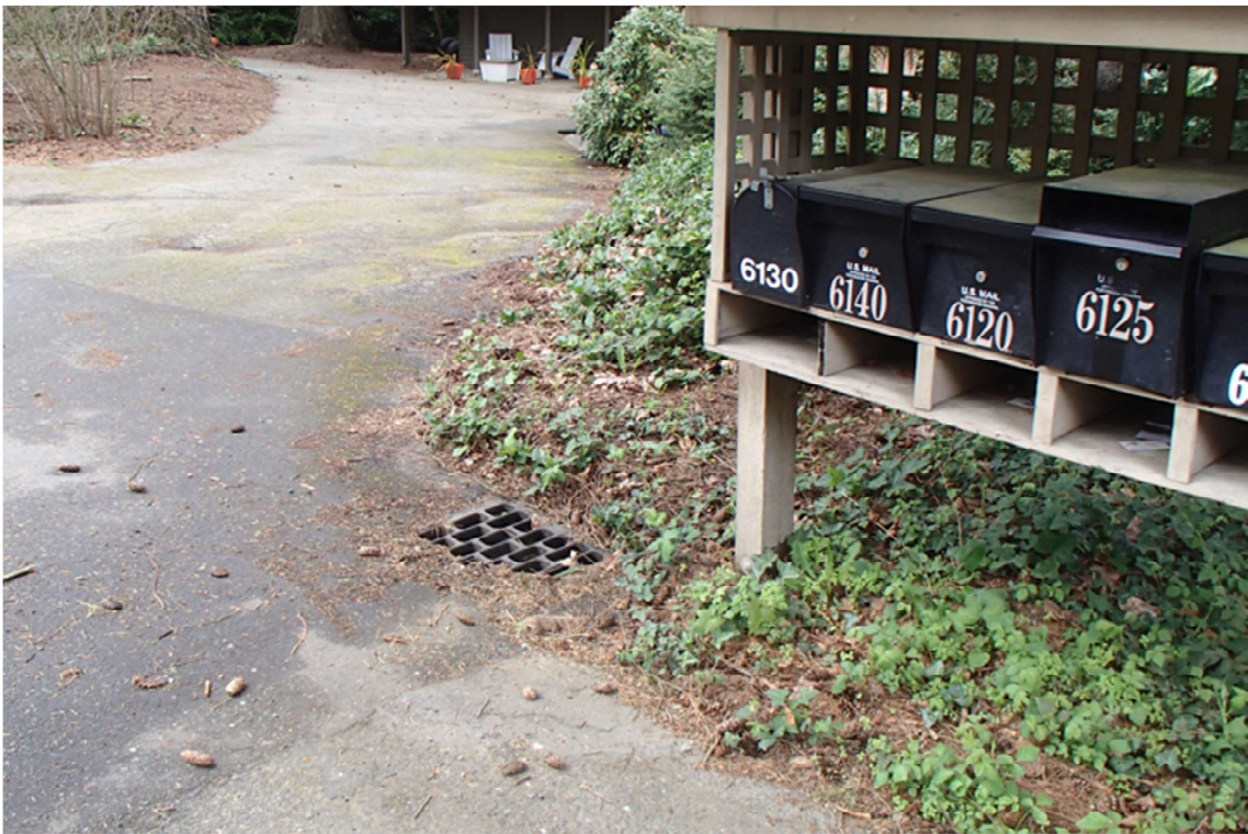
Photo No. 3 Looking northeast at CB 30a-9 between House #6130 and #6140
