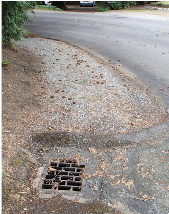
Photo No. 7 Looking southwesterly at CB30a-52 opposite House #6019 and #6017. Note gravel lip and vaned grate to catch runoff down steep road grade.
